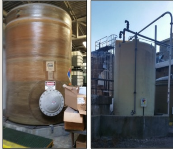
Justin FRP Tank on Brine Service (Left) and ASSMANN ICT 6500 Tank on HCl Service (Right)
